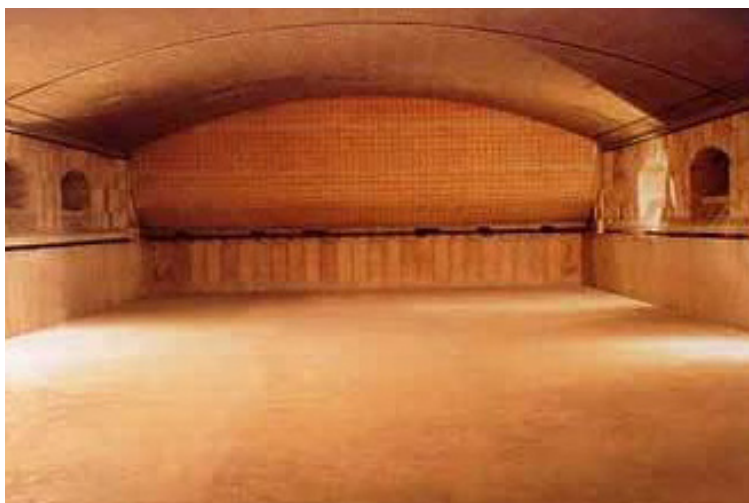
Figure 1. The interior of a glass furnace after a rebuild indicating undamaged refractory lining.
