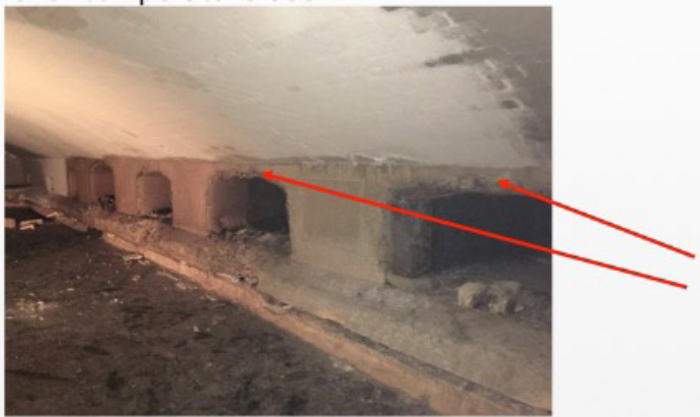
Figure 2. Damaged refractory around the ports is caused by over temperature use.
